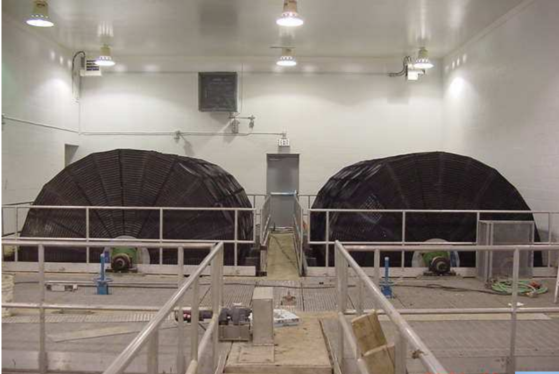
▲ NR-RBC – Wasbaseemoong First Nation. Ontario, Canada Design Flow: 2150m 3 per day
