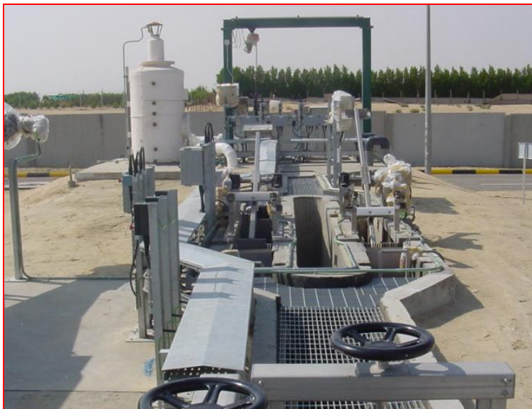
▲ NR- Mechanically Cleaned Arc Screen Installation – Al-Wafra Kuwait Design Flow: 4000 m 3 per day
