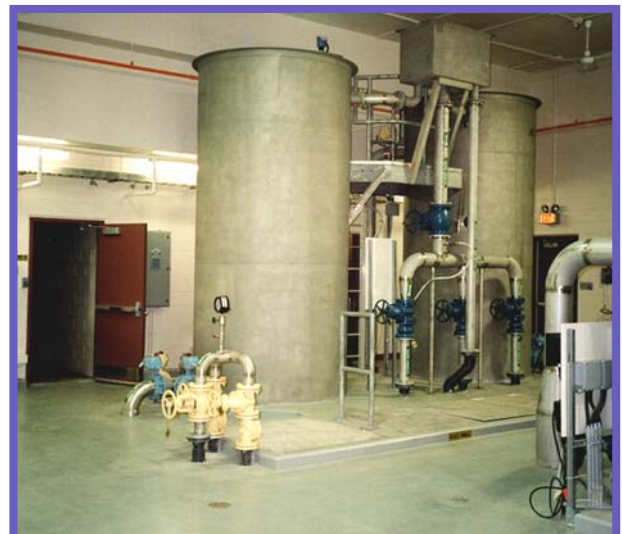
NR-GAC Tower, installed in 1999 at Echo Bay, Ontario, Canada, to remove organic contaminants
