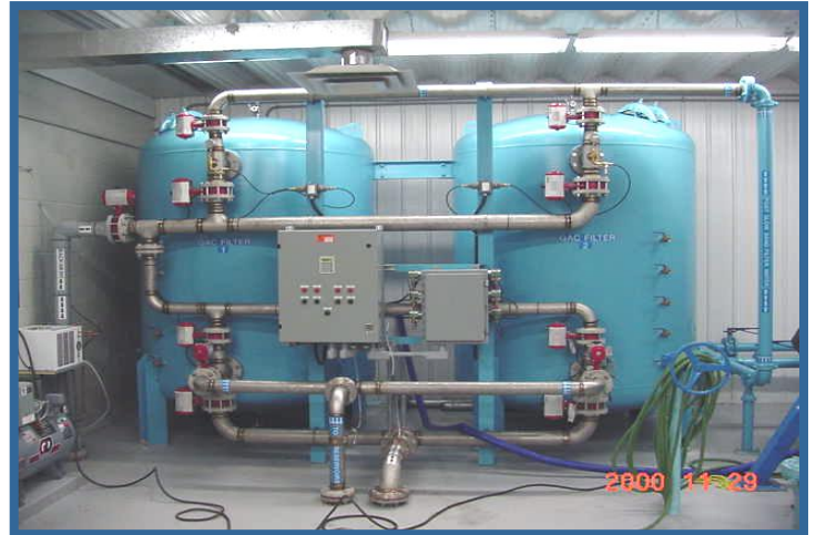
▲ NR-GAC Filter - North Caribou, First Nation, Ontario, Canada Design Flow 1080m 3 per day
