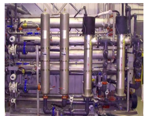
Nanofiltration System Ebb & Flow, Manitoba, Canada Design Flow: 1850m 3 /day
