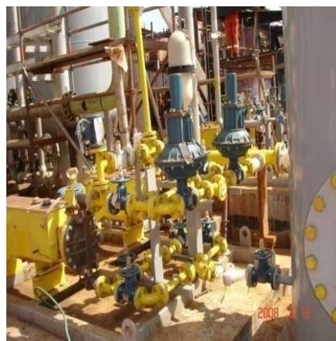
Chemical Regeneration Moa Nickel, Cuba Design Flow: 6720m 3 per day
