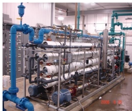
Nanofiltration System Rolling River, Manitoba, Canada Design Flow: 648m 3 /day
